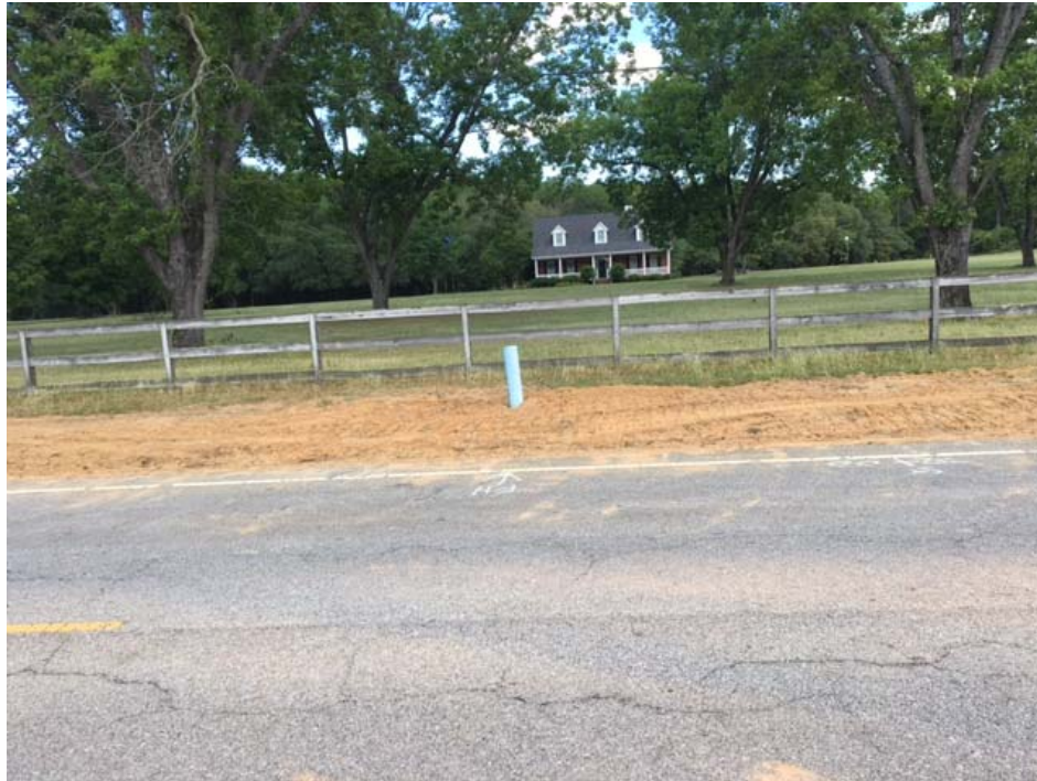
Photo 2: Fire hydrant stub Lower Richland Blvd
