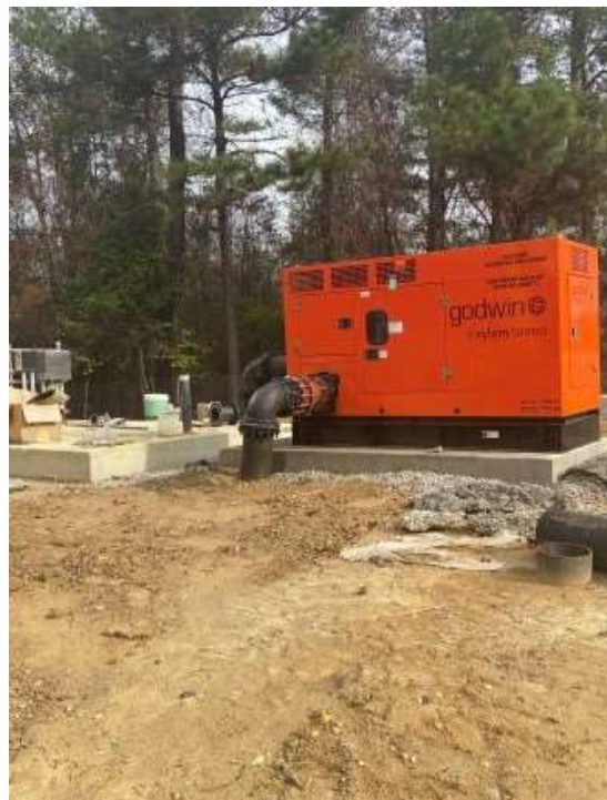
Photo 1: Garners Ferry bypass pump
