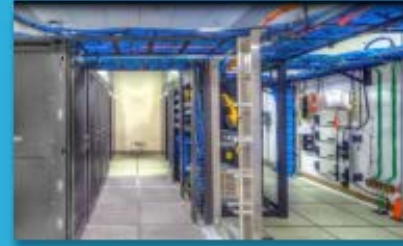
IT Server Room
