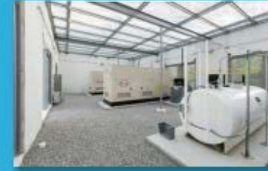
Fuel Storage / Generators
