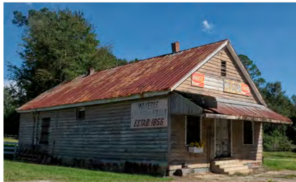
Preservation and adaptive reuse of the historic Wateree Store could help tell the story of mercantile culture in Lower Richland while providing goods and services for the resident and visitor communities.
