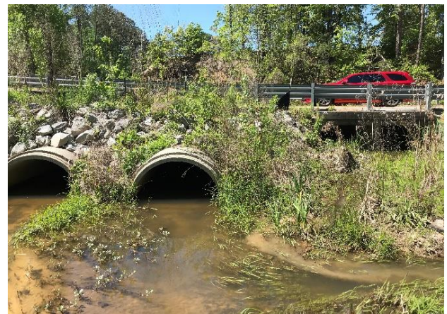
Figure 6. New 60" RCPs at repaired crossing of Spears Creek Church Road. Note sediment deposition in older box culverts under car at right and side channel at bottom right. View is upstream from the east side of roadway.
