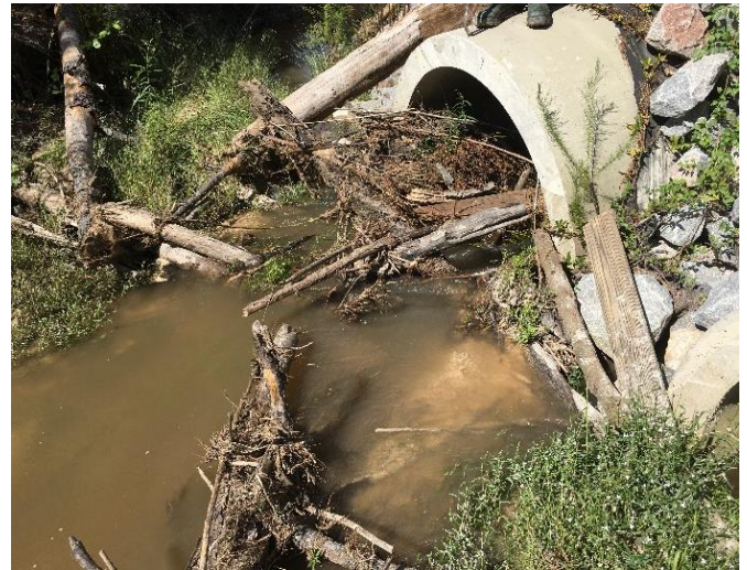
Figure 11. Sediment and debris blocking culvert upstream of Spears Creek Church Road .
